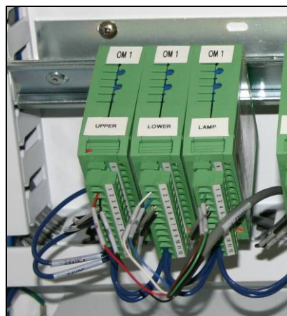
Figure 17: Multiple Monitors, each with a connection to a separate Compact Sensor™
